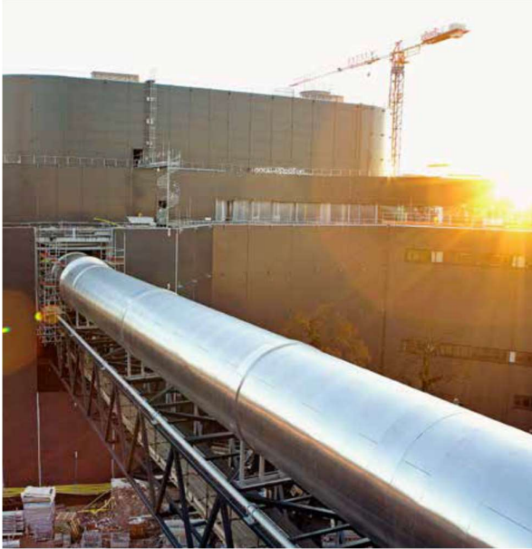
Figure 1: Stockholm’s combined heat and power (CHP) plant contributes to Stockholm’s goal of being a fossil-fuel-free city by 2050.
